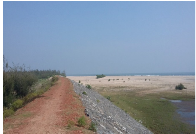
Geo-synthetic embankment wall at Padmapur, constructed by the Odisha government with support from the World Bank.
